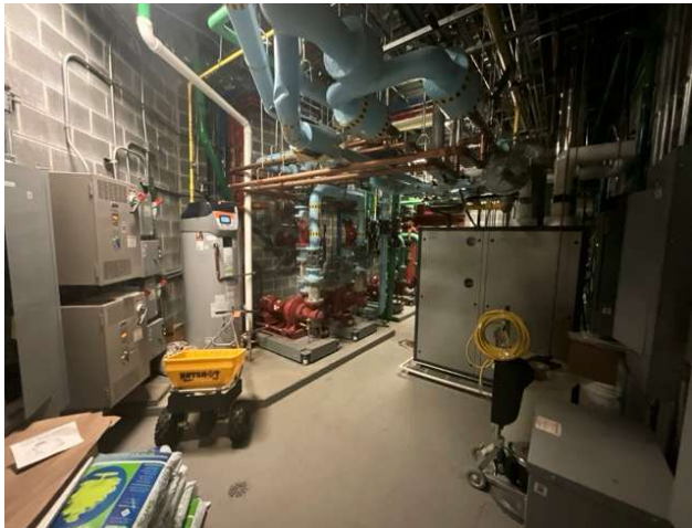
21 - NEW BOILER ROOM
