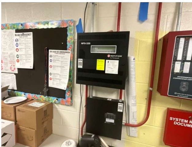
23 - FIRE ALARM PANEL
